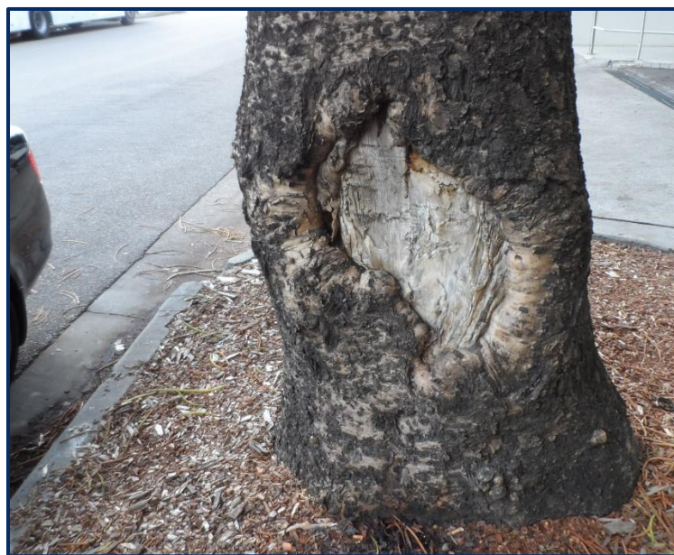
Figure 7: Mechanical damage to buttresses.
